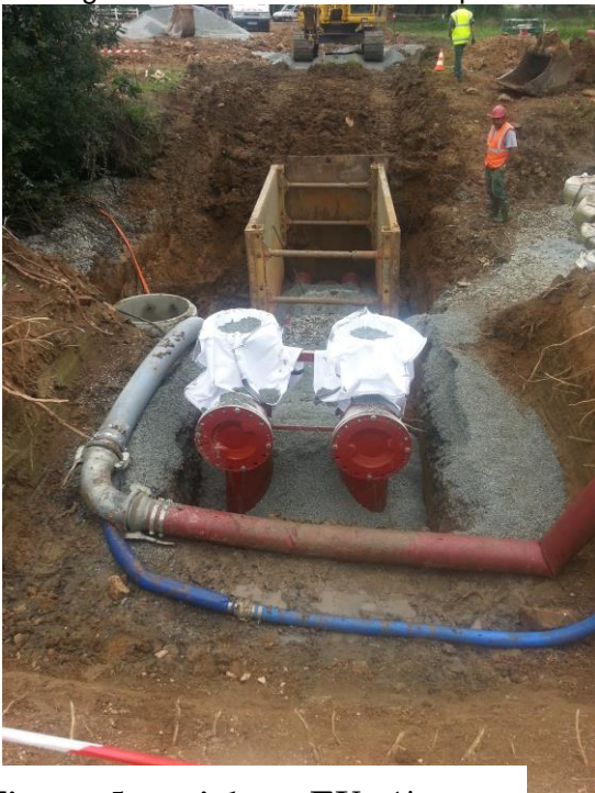
Figure 5 : siphon EU (Antes – Niort)
